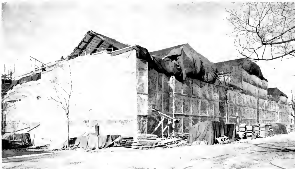
EVEN IN SUB-ZERO WEATHER, bricklayers could work inside the novel "plastic wrapping." The covering, believed one of the largest anywhere, provided a steam-heated corridor on the outside of the Quodrangle. View is from the southeast.
